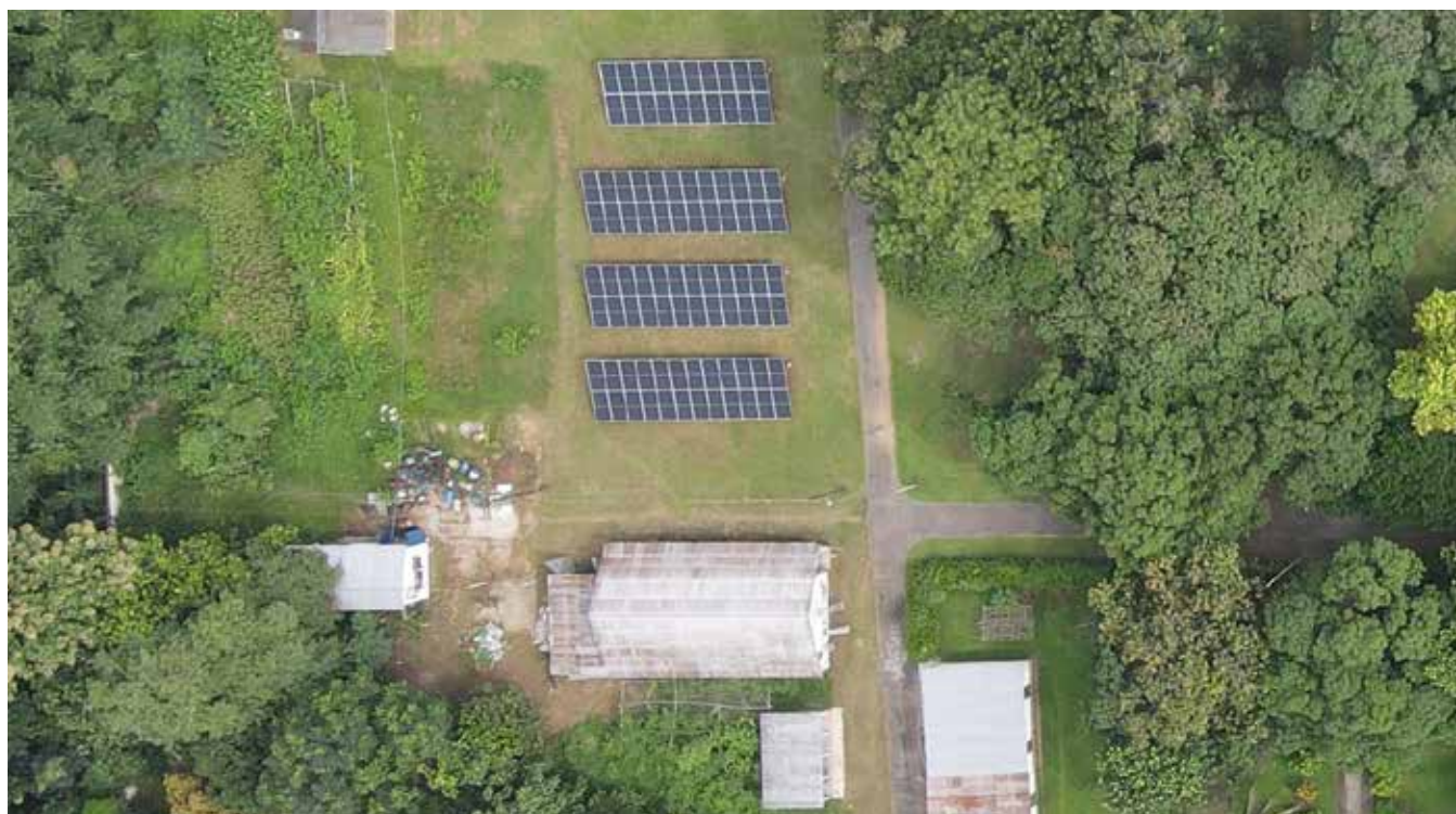
Solar Power Plant at Jalchatra Hospital
